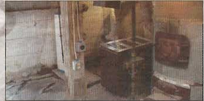
NEARLY DONE: Shoddy workmanship can be a real problem
